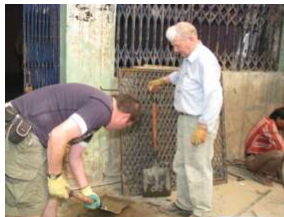
Members of Ballymena Builders team, Northern Ireland rebuild the Asha centre in Dr Ambedkar slum
